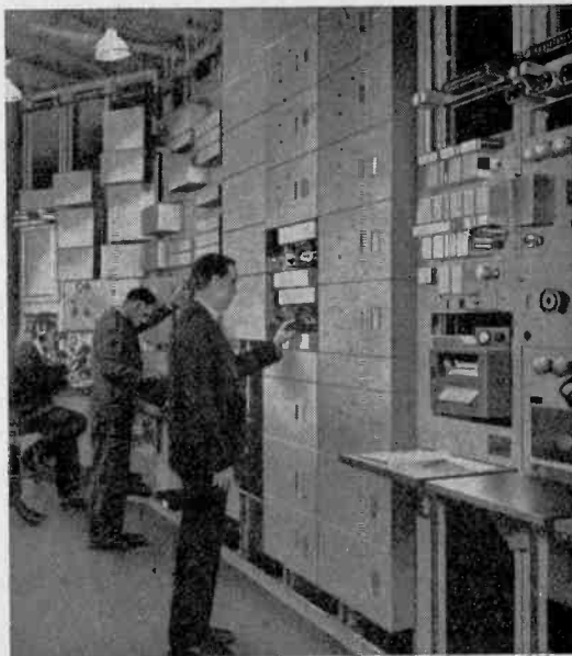
Fig. 4. New York terminus of carrier telephone system.
